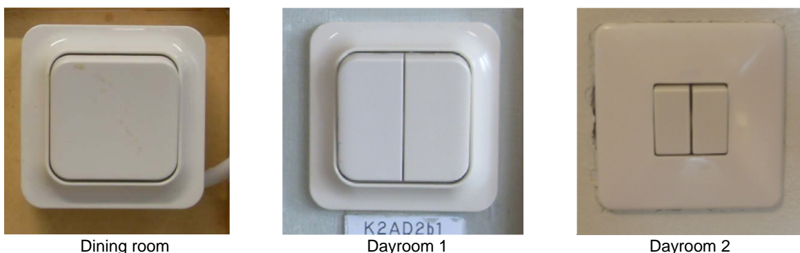
Figure 3 Lighting control devices in the rooms
